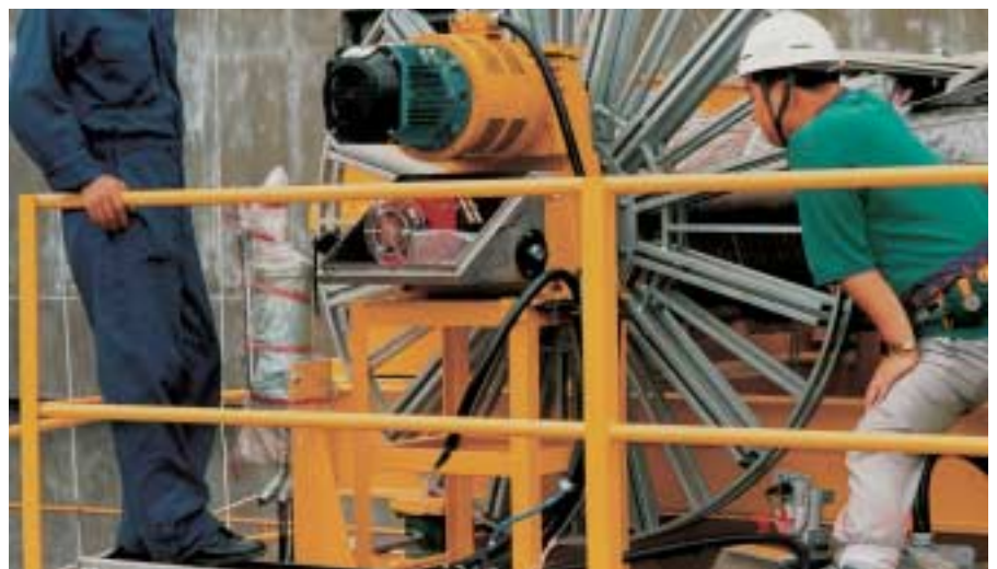
A cable reel being commissioned in Korea for a compost plant application.
