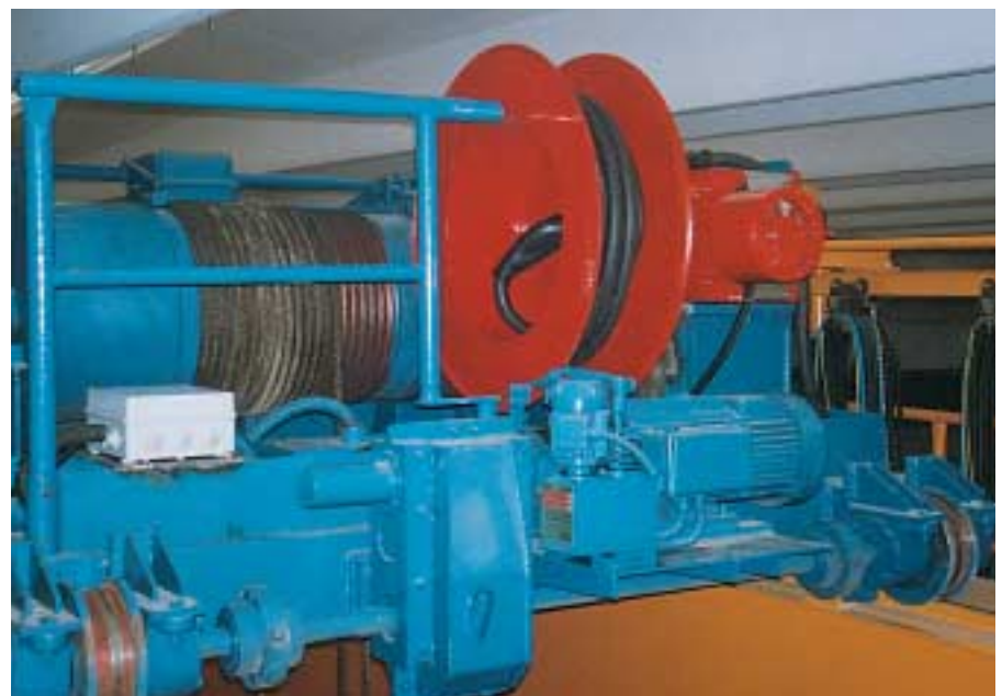
A vertical reel application at work in a steel mill.
