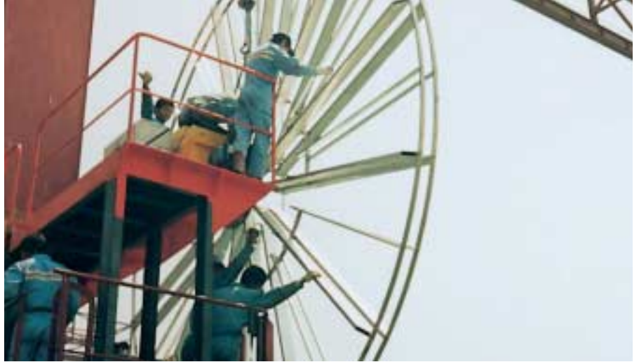
One of our drums during erection in a harbour application in Singapore.
