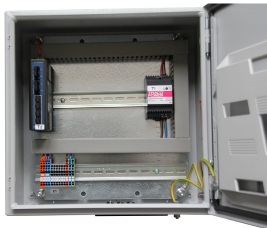
Figure 10: Fibre Optic Converter Box
