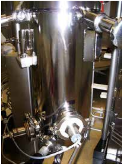
Fig. 1: Level control in a container with non flush mountable sensors
